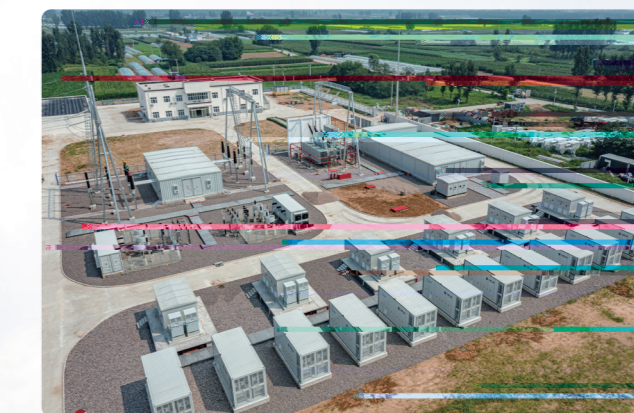
BESS Power Station
